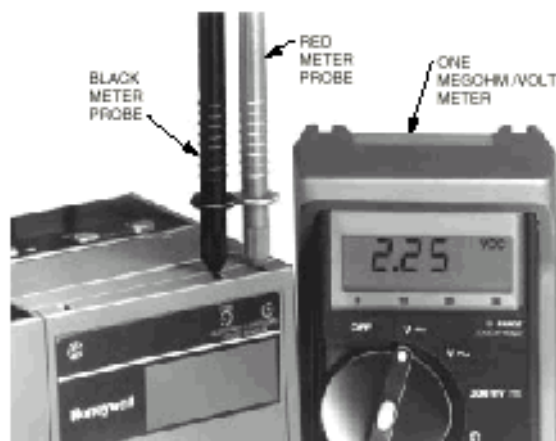
Fig. 13. Measuring voltage flame signal with 7800 SERIES controls.
